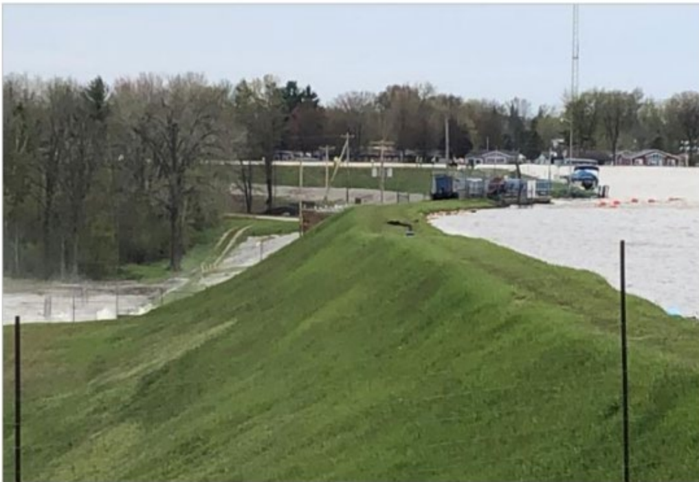
Figure 3-4: Photograph Showing the Downstream Side of the Edenville Left Embankment at 5:31 P.M., Tuesday, May 19, 2020
