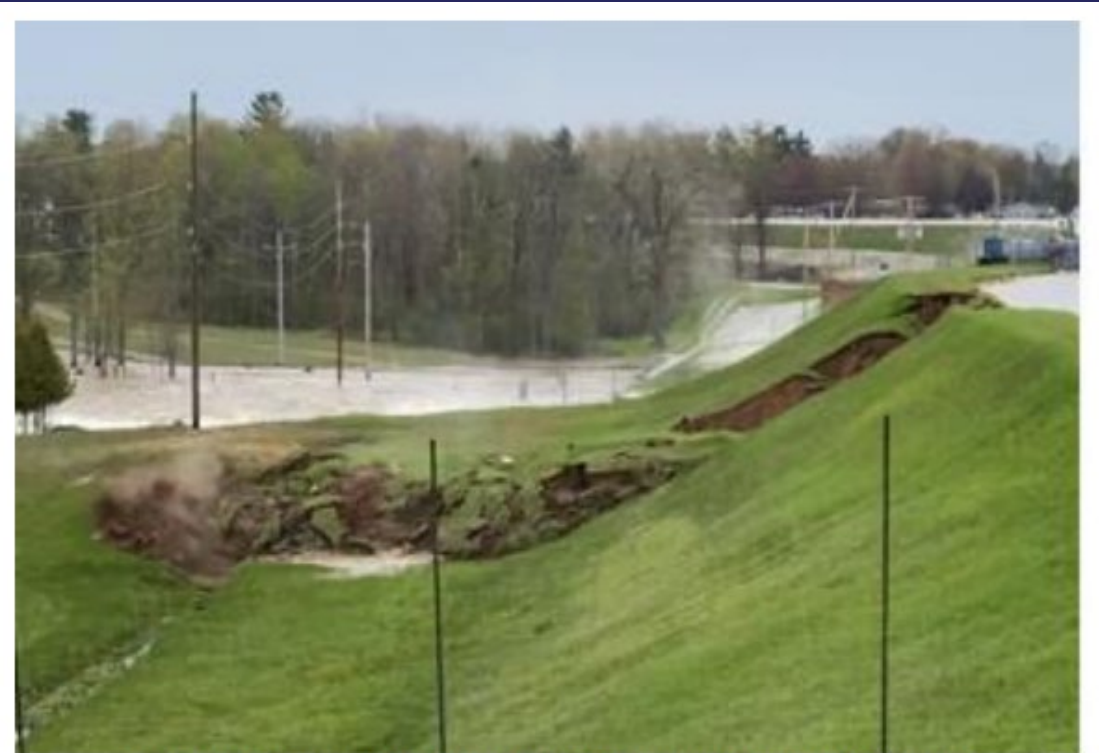
Figure 3-11: Enlarged Still Image from Dam Failure Video at 10 Seconds
