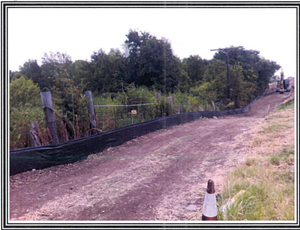
1. View northeast from the western limit of the new 18" diameter wastewater line along FM 3406 in Round Rock, Texas.
