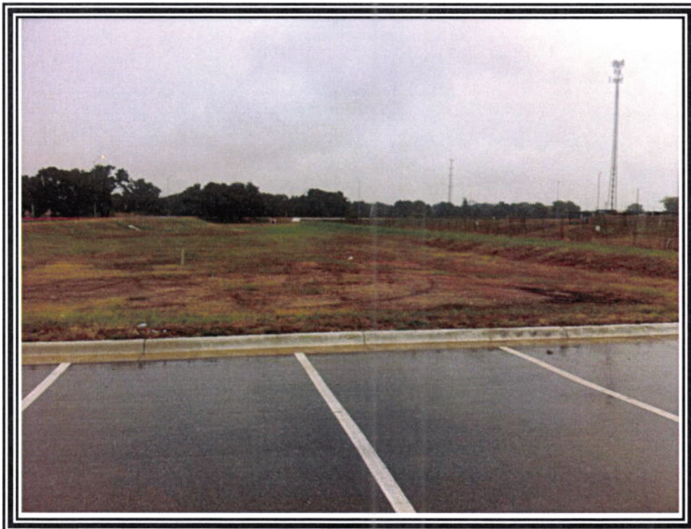
12. View northeast along the north wastewater line from just south of detention pond feature S-1.
